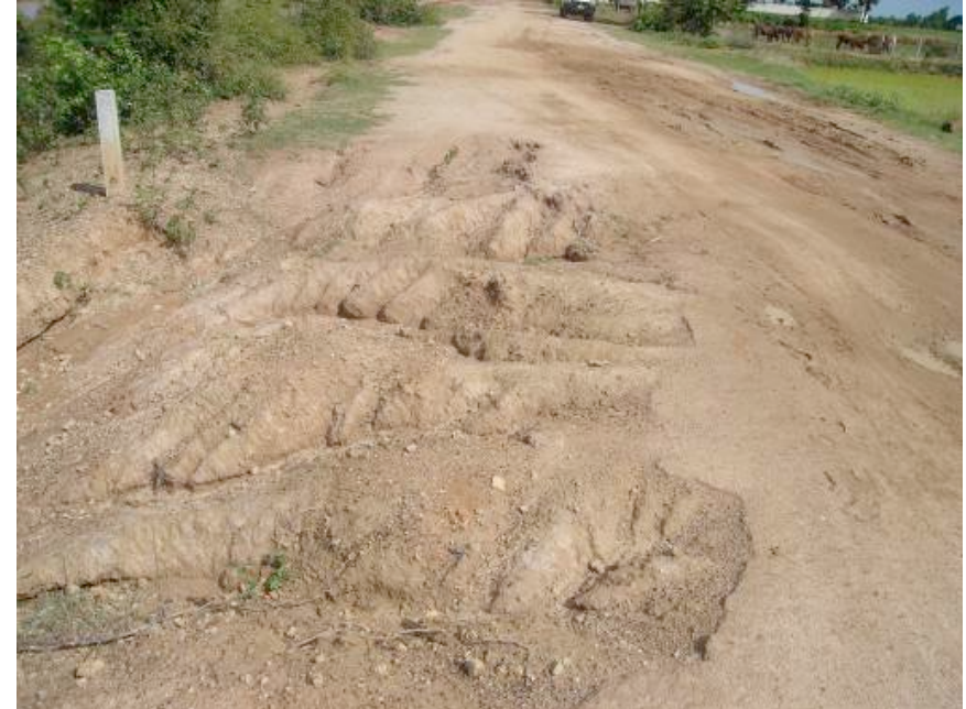
Damage to rural road by flood
